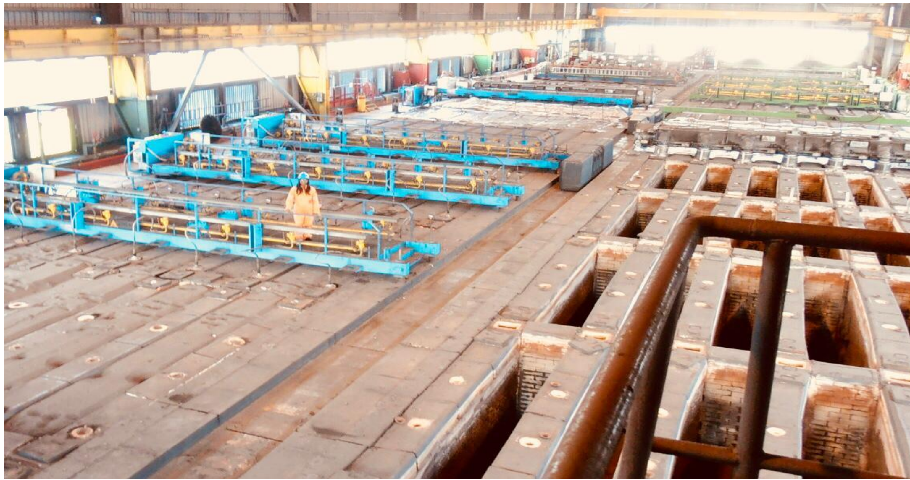
Figure 1. Anode baking furnace at Aluchemie, Rotterdam
