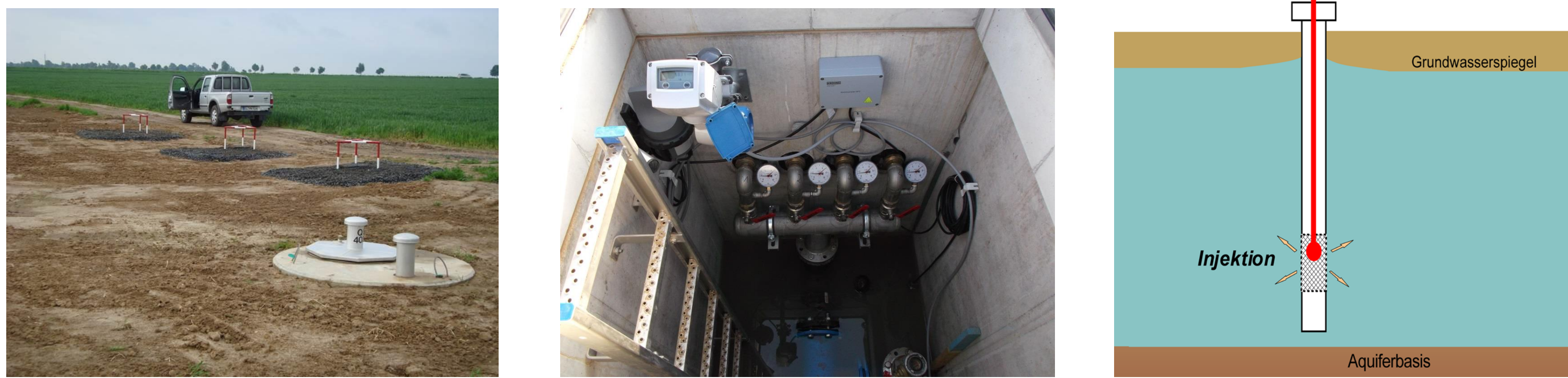
Figure 1. Injection (recharge) well; ground view (left), look inside top (center), scheme (right)
